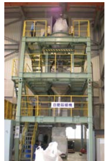
Automatic sampling equipment
