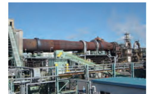
Rotary kiln incinerator at JX Nippon Tomakomai Chemical Co., Ltd.
