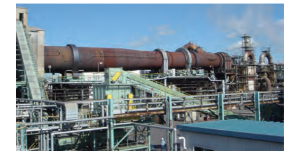
Rotary kiln incinerator at JX Metals Tomakomai Chemical Co., Ltd.
