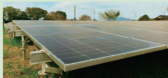
Example of a solar power generation system installed by a PPA operator
